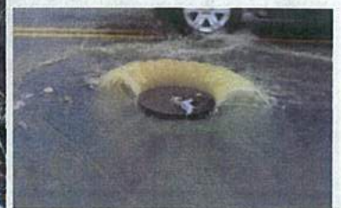
Raw Sewage runoff
